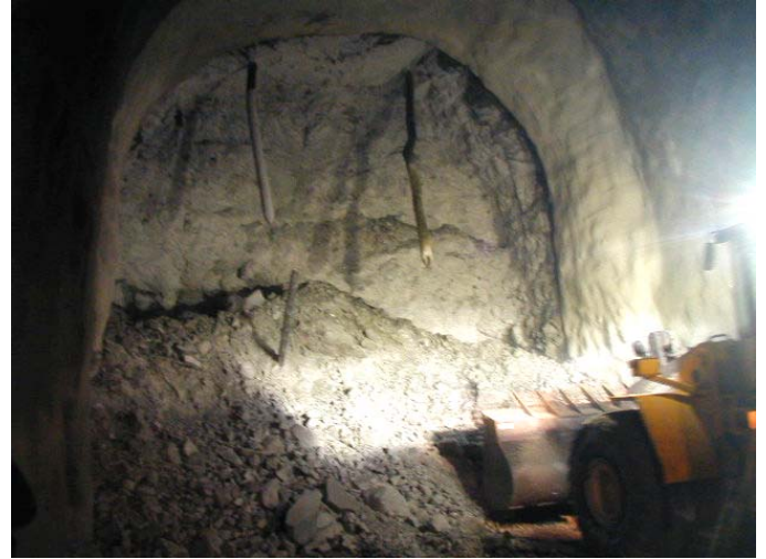
Fig. 9. Tunnel end after blasting. The cooling pipes for tunnel soil freezing were emptied before blasting.
