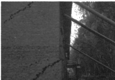
Fig. 1 Two Storied-Building Damaged in South Yunnan
