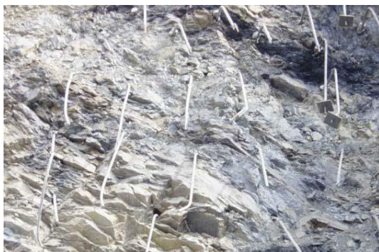
Fig.7. Northern unsuccessful soil nailing project
