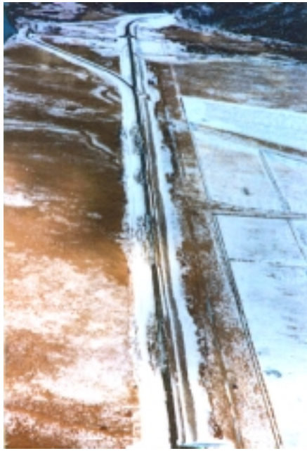
Fig. 2. Aerial photograph of the damaged dike
