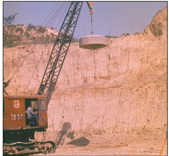
Photo 1. Heavy tamping of the excavation bottom - L 1 , FS 1 , L 2 and FS 2 can be distinguished on the vertical slope
