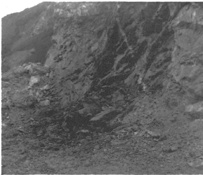
Fig. 3 Photo showing rock slide
