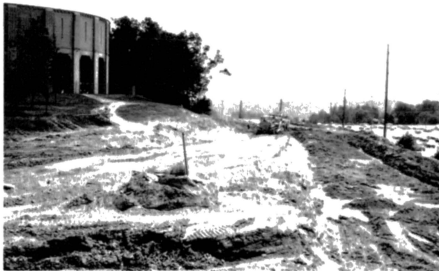
Fig. 9. Construction Excavation Problems
