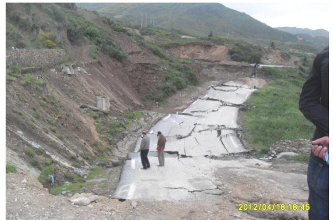
Fig. 8. Overview of landslide Assoumeth RN24, PK 226+300.
