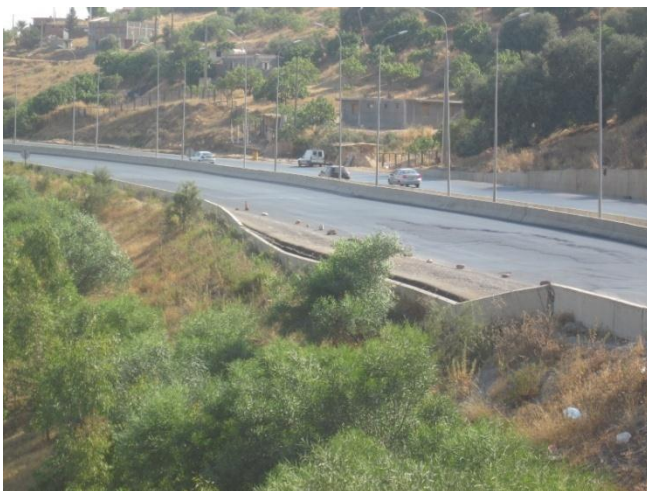
Fig. 3. Landslide at Ain -Tork, Department of Bouira, East-West highway A1, April 2012.
