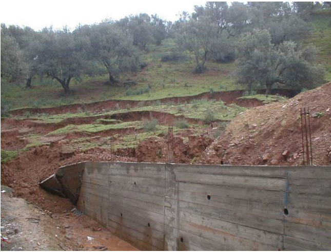
Fig. 1. Landslide at Beni Amrane , Department of Boumerdes, causing damage to retaining wall, January 2003.
