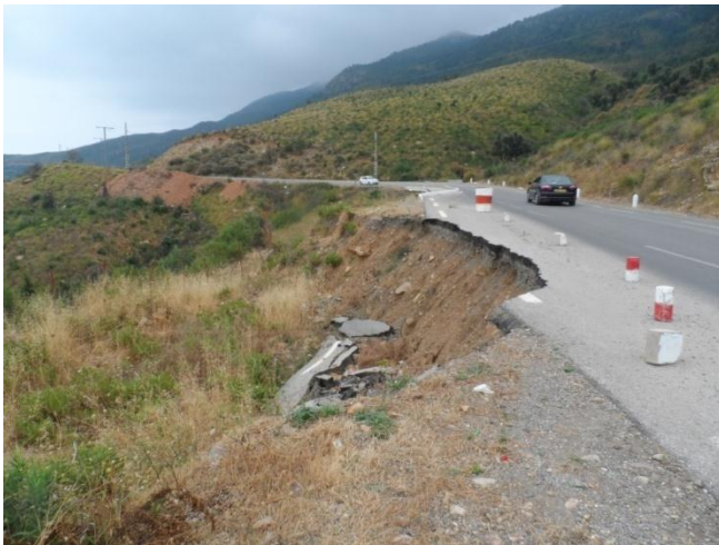
Fig. 2. Landslide at PK 227+110, RN 24, Bejaia, 2011.
