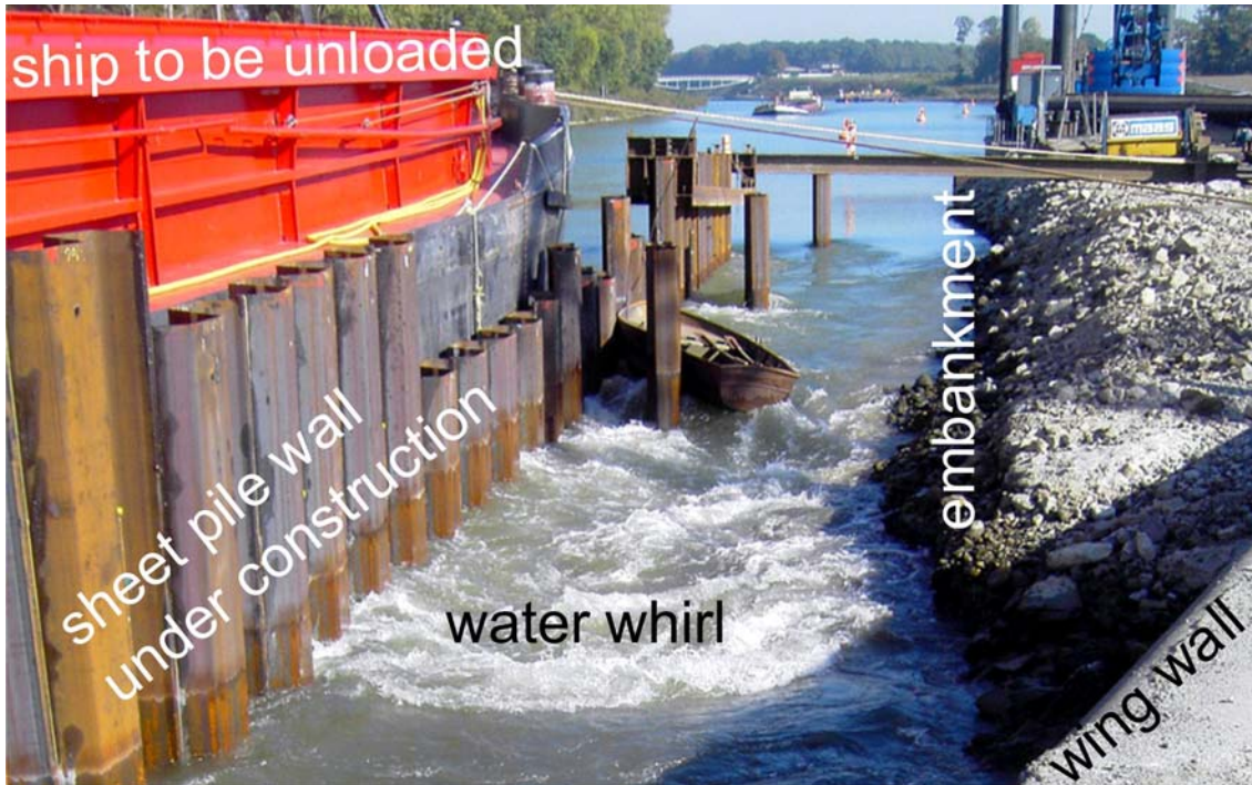
Fig. 3: Water whirl in front of the wing wall of the northern abutment
