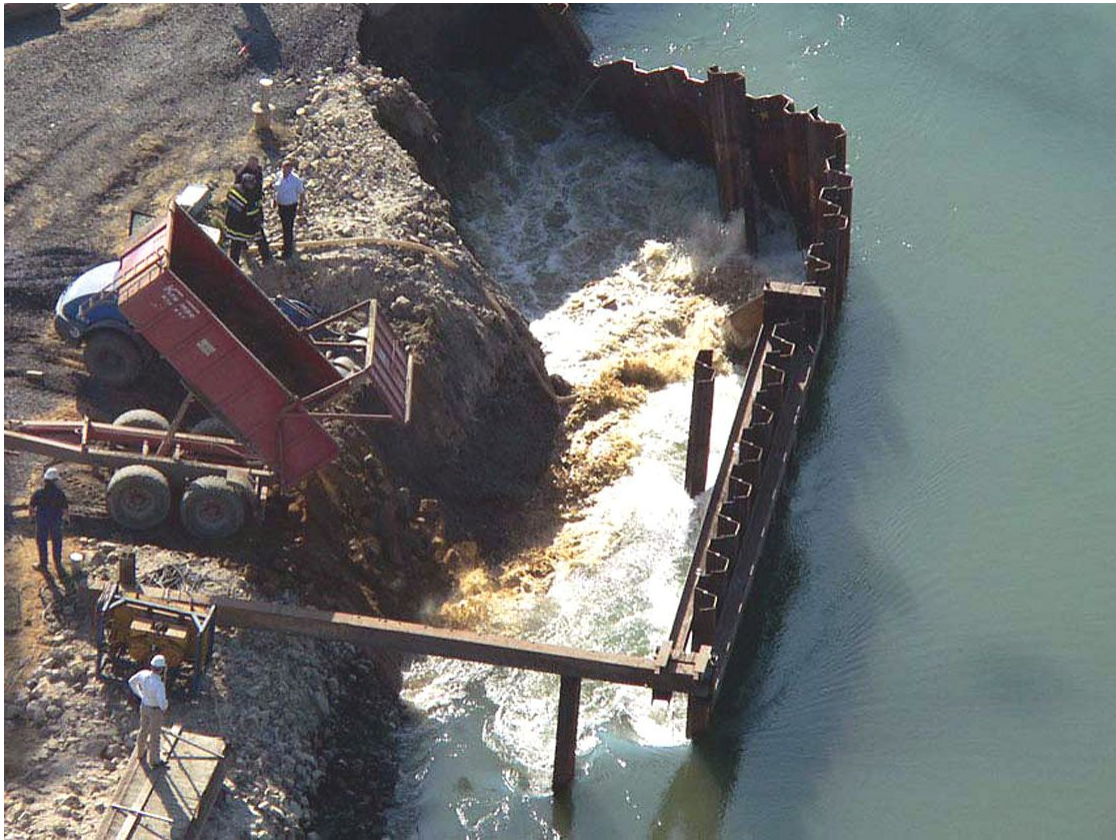
Fig. 7: Attempt to close the leak by dumping soil material into the canal
