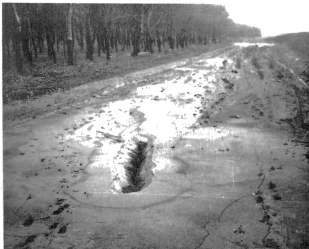
Fig. 6. Ejected sand near levees
