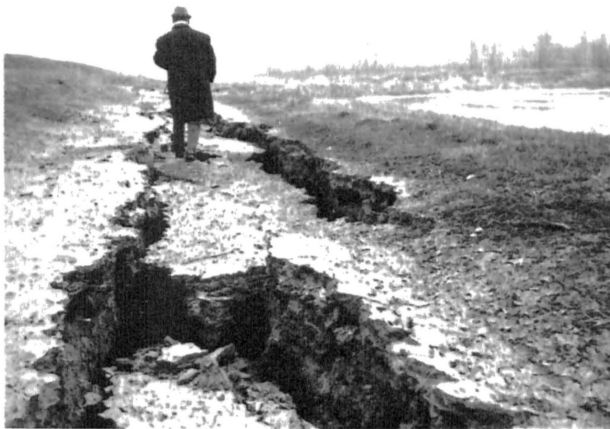
Fig. 5. Longitudinal cracks observed on levees
