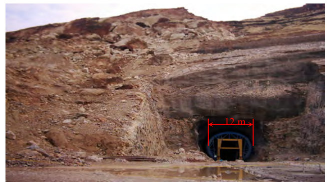
Fig. 10. The view of power tunnel intake and unstable rock blocks in the above after intensive rainfall leading to final collapse
