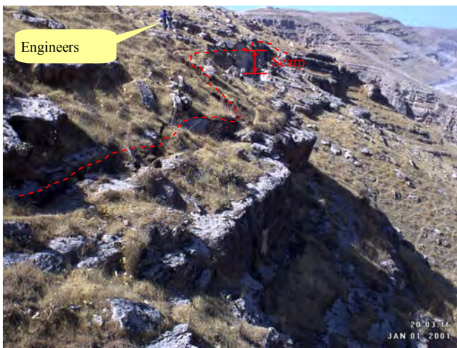
Fig. 8. Trace of main tension joint of the sliding mass on ground surface and resulting scarp
