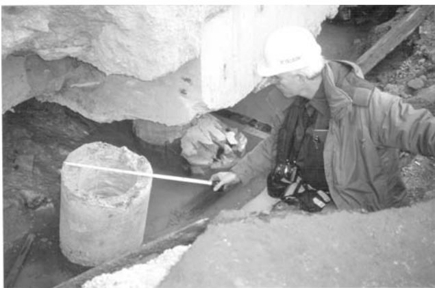
Fig.3. Shearing of a pile by ground displacements in 1995 Kobe earthquake (Finn and Fujita 2002).
