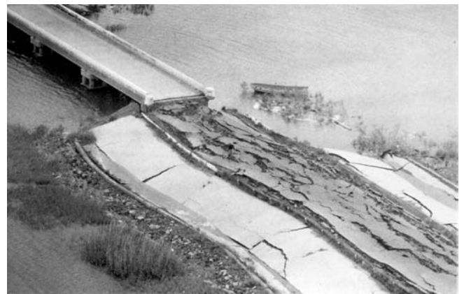
Fig.4. Bridge on undamaged pile foundations with failed approaches due to liquefaction (Finn and Fujita 2002).
