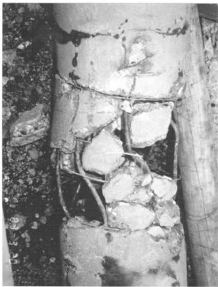
Fig.2. Damage to pile by 2m of lateral ground displacement during 1964 Niigata earthquake (Yoshida et al. 1990).
