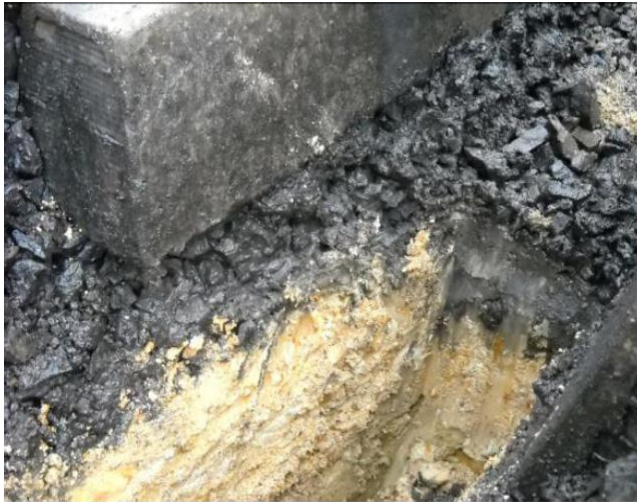
Fig. 5. Ballast fouling due to coal and subgrade pumping (Photo courtesy of Michael Martin, QR National)
