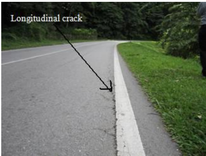
Fig. 16. Longitudinal crack was observed parallel to the edge line of the road
