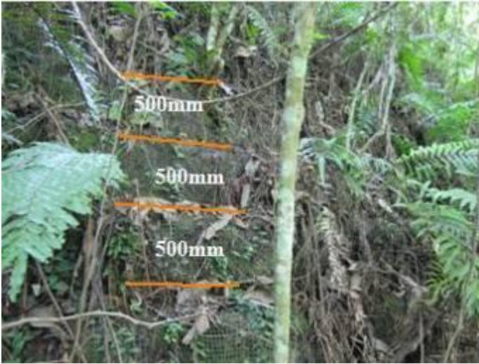
Fig.19. Photo taken on September 11, 2012 shows layers of full layer thickness (500mm) of geogrid facing
