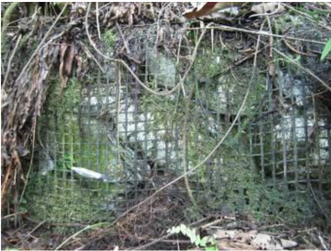
Fig. 20. Photo taken on September 11, 2012 shows geogrid facing clearly intact 15 years after it was constructed
