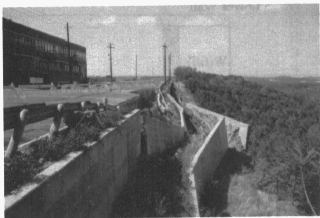
Fig. 2 View of the Failed Section of Wall
