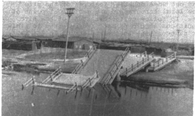
Fig.3 Plate girders of highway bridge thrown and overlapped longitudinally whereas nearby warehouses stood still
