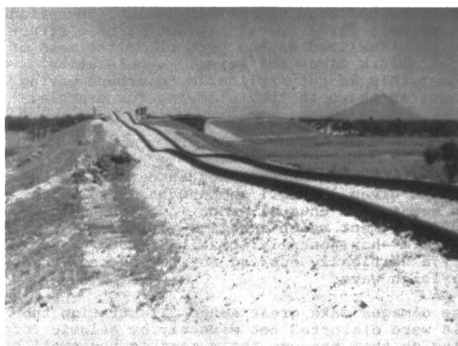
Fig.2 Rails rocked purely vertically due to Rayleigh wave action (Tangshan event M=7.8, 1976)
