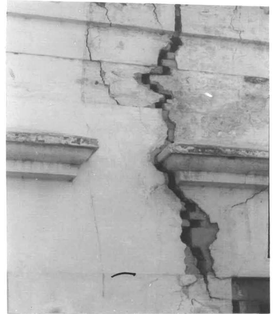
Fig. 4 Severe Cracking near Lintel
