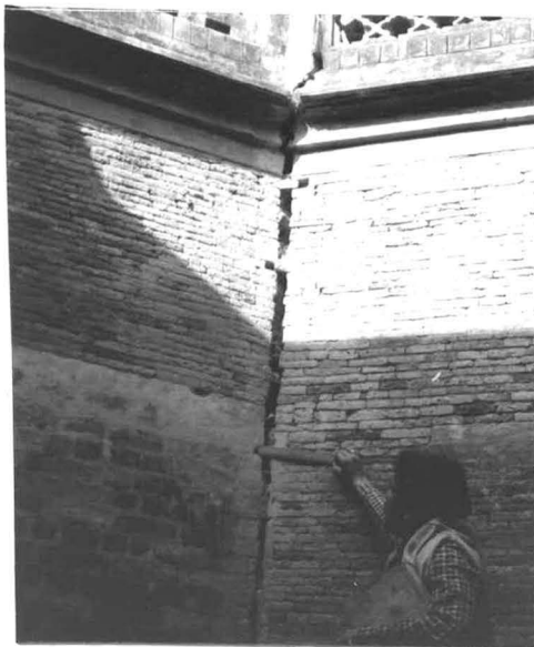
Fig. 3 Separation of Walls at Corner
