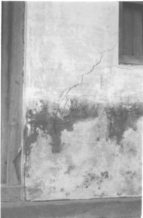
Fig. 8 Cracks in newly constructed building showing seepage in wall
