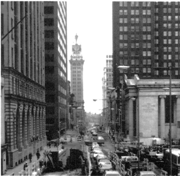
Figure 2. View looking east along Baltimore Street during construction of Charles Center Metro Station.
