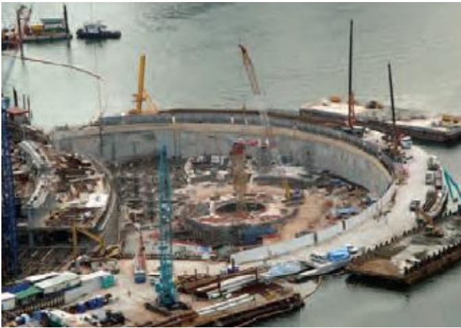
Fig. 5. Areal view of excavation inside a 120m cofferdam and the 130m semi circular cofferdam.
