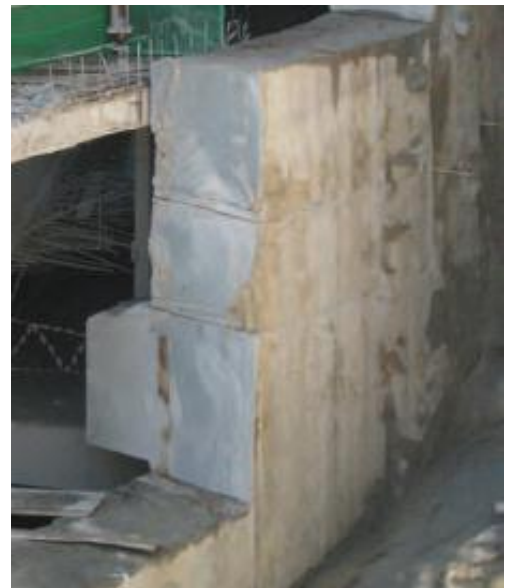
Fig. 9. Locations of wall removal (in red) and cutting of the diaphragm wall exposed above excavation level.
