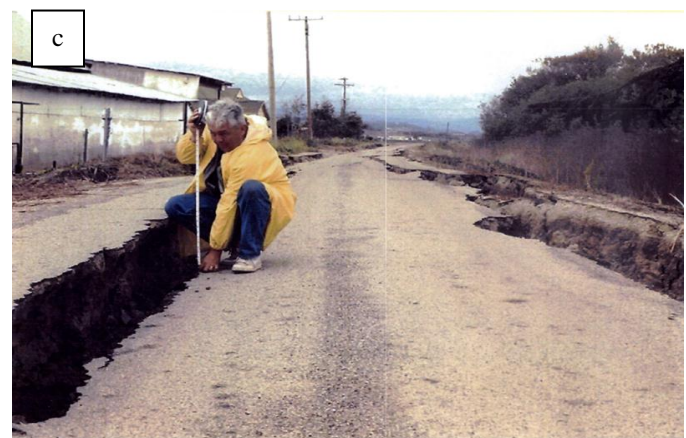
Fig. 3. Excerpts from the US Army Corps of Engineers Memo for Record dated 23 October 1989 (author: David Ricketts): a. Map of inspected damaged levee; b. Typical cracks and slumping of levee; c. Most damaged location.
