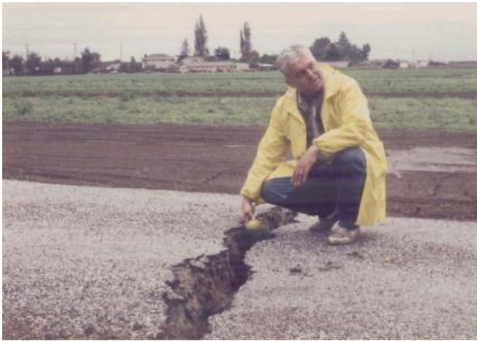
Fig. 4. Transverse crack through entire levee section (photo David Ricketts).
