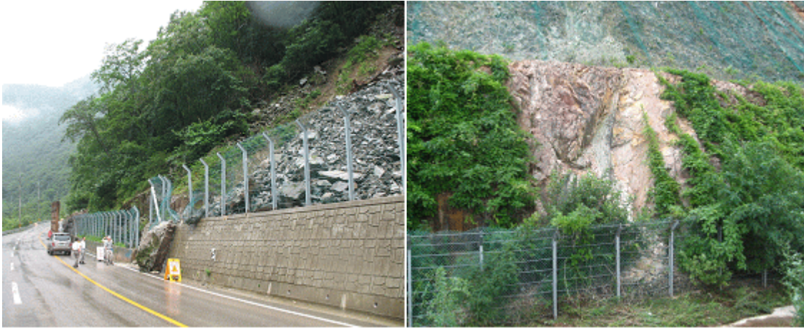
Fig 4. The Damage Example due to Stone falling
