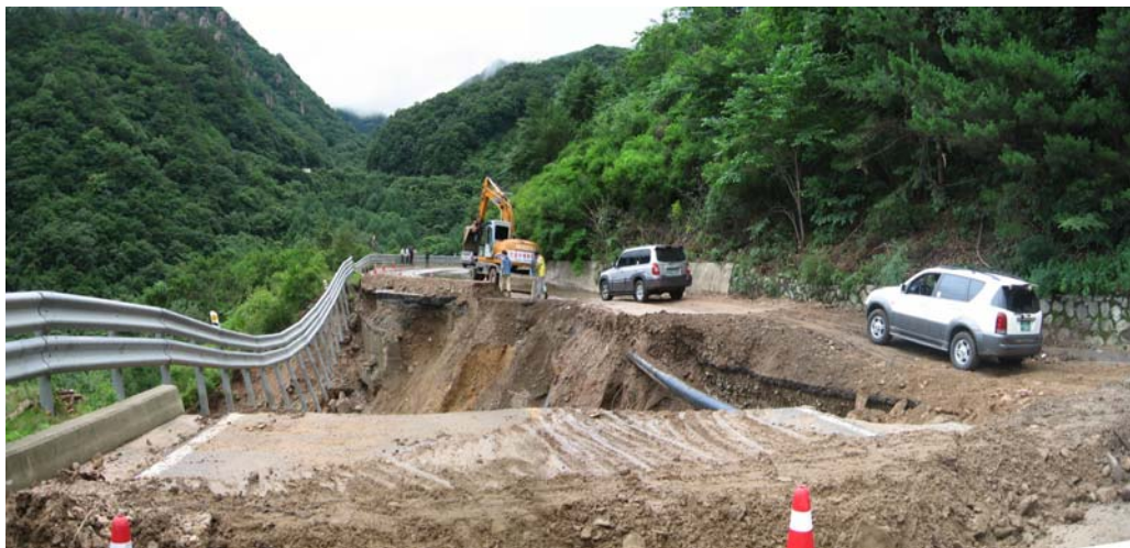
Fig 9. The damage example by banking section
