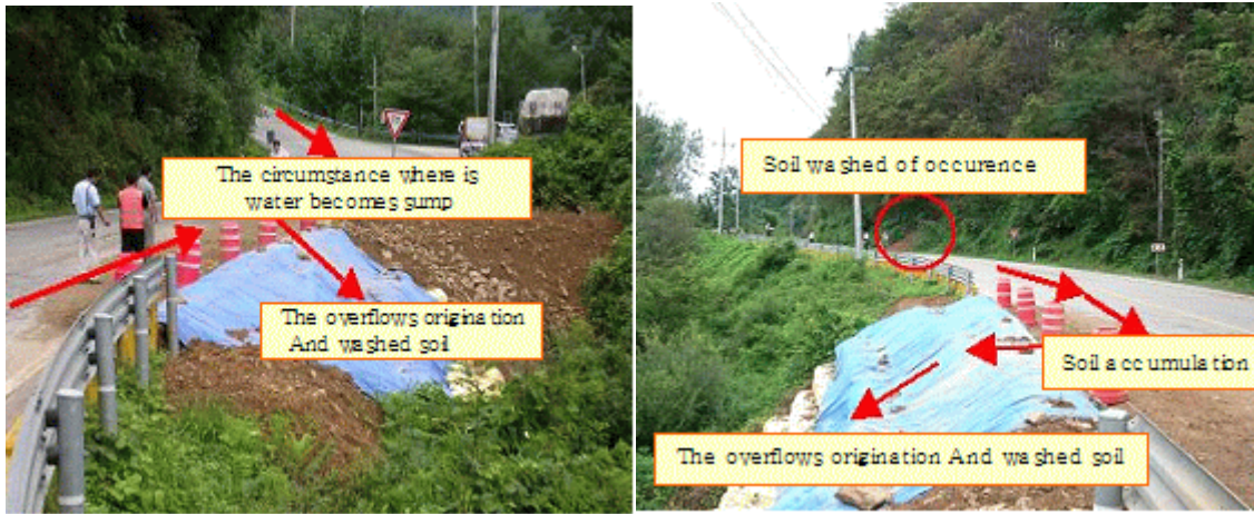
Fig 10. The damage example due to washing of fill material
