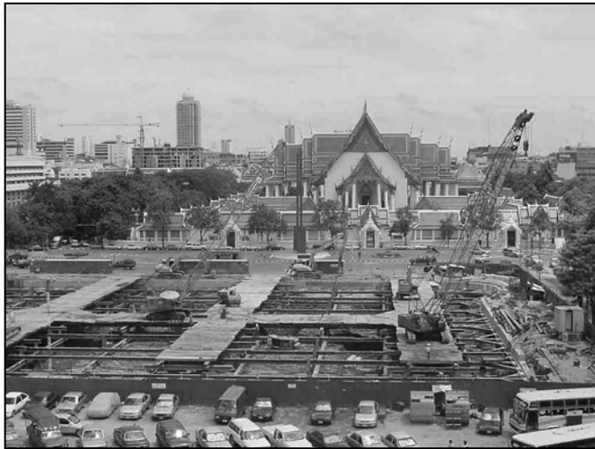
Fig. 9. Phase 1 excavation work in progress with historical Buddhist temple Wat Suthat in background (Phase 2 area was being used as car parking space)
