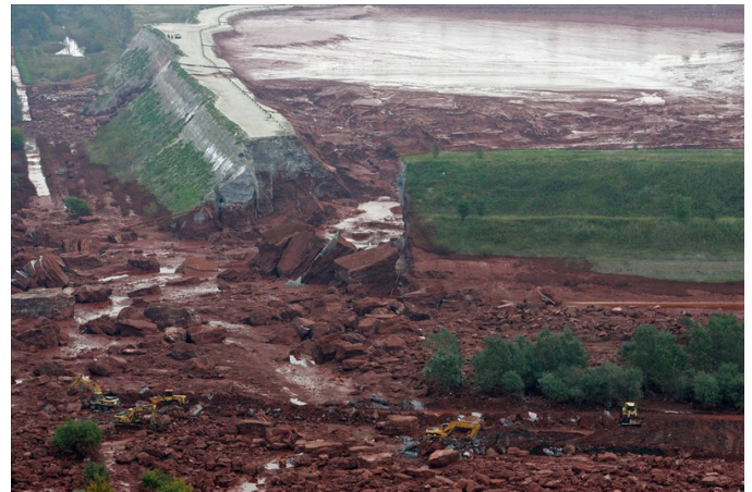
Fig.23. The cracked dam corner
