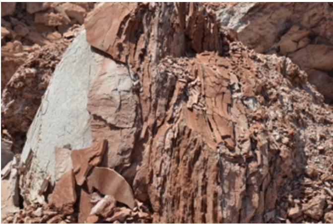
Fig. 7. Dam section by the rupture
