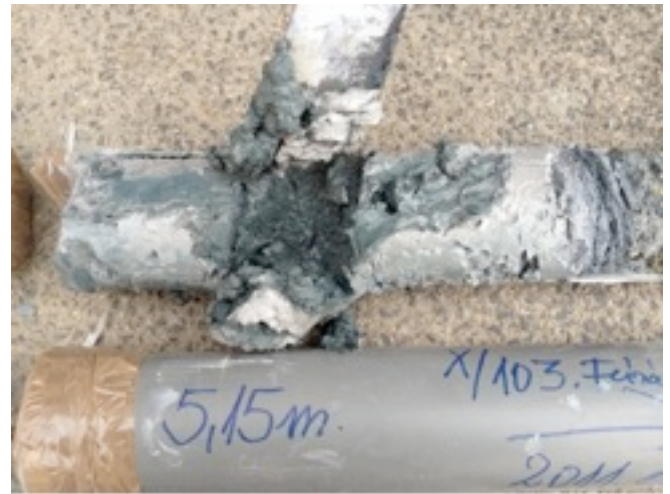
Fig. 9. Completely soft dam part
