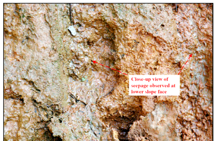
Figure 12. Close-up view of observed seepage at the face of the slope.
