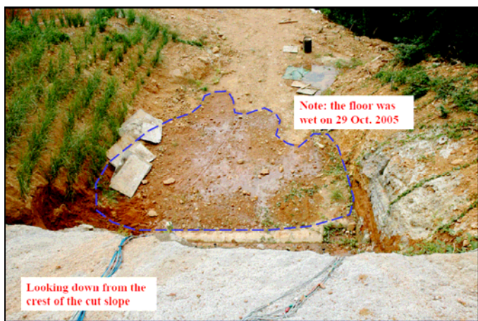
Figure 13. The floor of the slope was wet on 29 October 2005.
