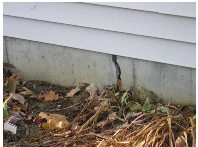
Fig. 2. Basement Wall Crack on North Side.
