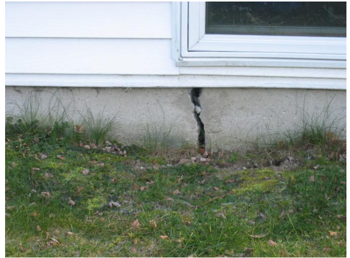
Fig. 1. Basement Wall Crack on South Side.
