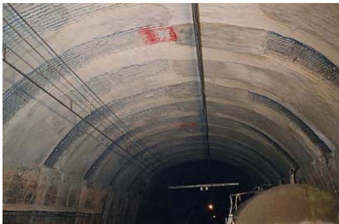
Fig. 10: Cutting the existing liner and installing the reinforcing support in alternating panels
