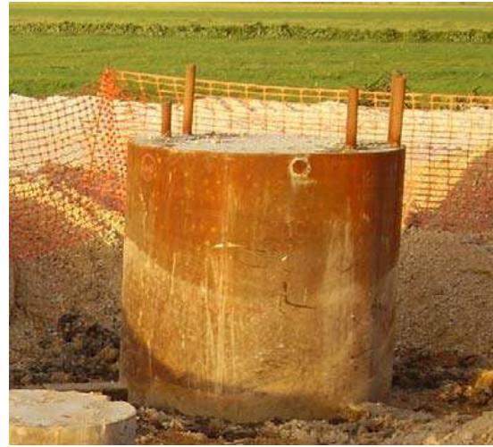
Fig. 50. 4 tubes for crosshole tests in a 1.5m diameter pile (after Ferreira et al, 2008)
