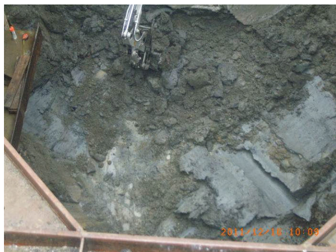
Fig. 7. Excavation Photographs below third row of bracing (a) South headwall (b) North headwall
