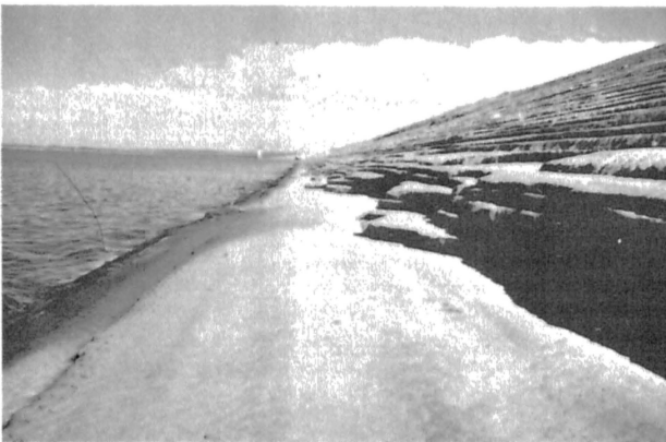
Figure 2. - View of most severely damaged soil-cement at Cheney Dam.
