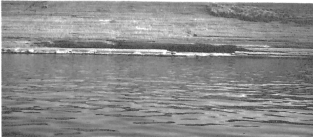
Figure 1. - Damage to soil-cement at Cheney Dam.
