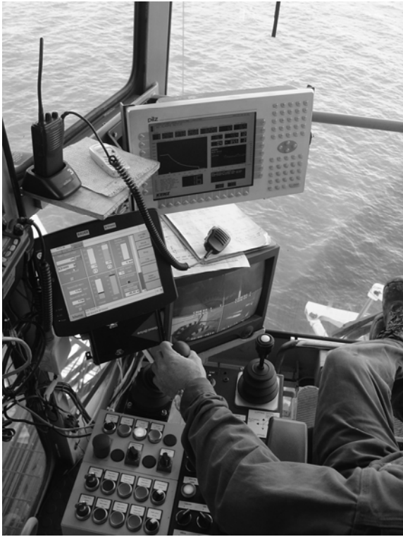
Fig. 16. B-Tronic monitoring, control and recording system inside crane dab
