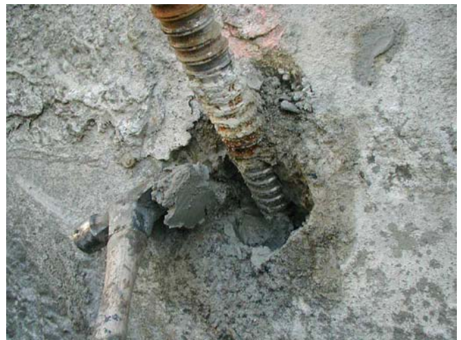
Fig. 10. Observed strut nail connection at existing wall.
