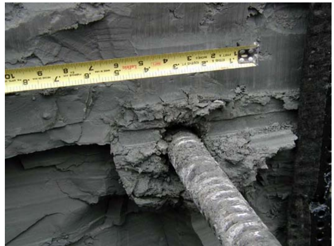
Fig 12. Nail hole annulus with no grout in drill hole or around nail bar
