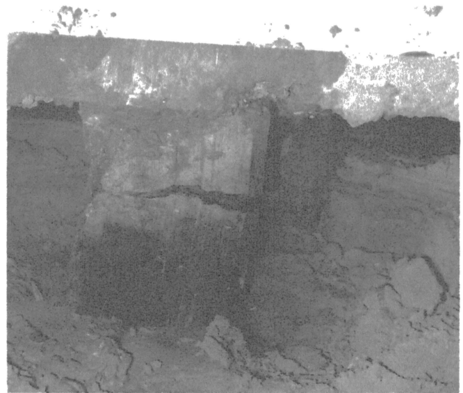
Fig. 8 A cracked concrete pile
