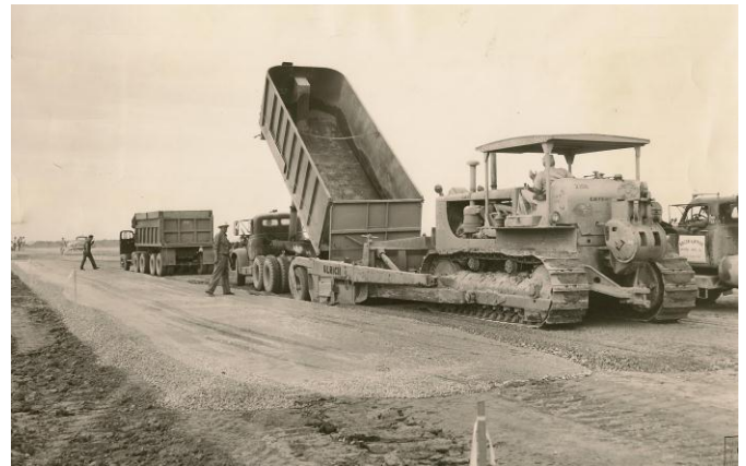
Fig. 42. Laying down aggregate base rock for one of the runway expansions at Chicago's O'Hare Airport (from Chicago Sun Times).
