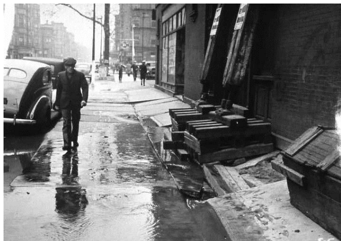
Fig. 27. Settlement of sidewalk induced by subway construction along the S-5 section of the State Street Line, between Grand Ave. and one block south of Division St. (Peck Collection-NGI).
