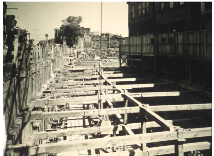
Fig. 37. Braced open cut on Contract S-1A of the Chicago Subway. This view was taken in July 1940 and shows the transition between the elevated and below ground sections of the State Street line, towards its north end, near the intersection with Clybourn Ave. (Peck Collection-NGI)
