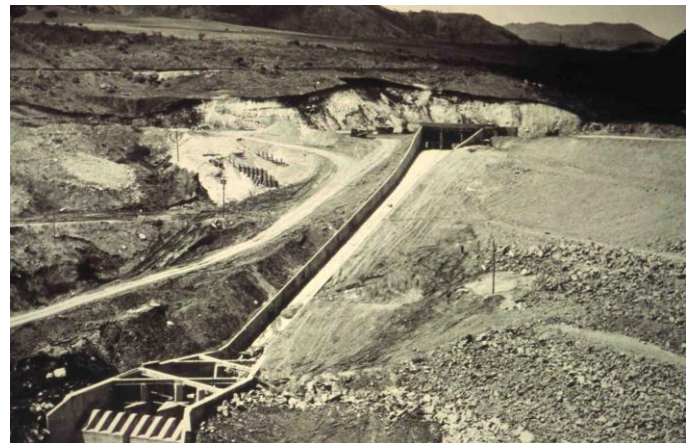
Fig. 24. Spillway chute and right abutment of Neusa Dam near Bogota, Columbia. The embankment was comprised of halloysitic clay laid on a thick mantle of landslide debris (Peck Collection-NGI).
