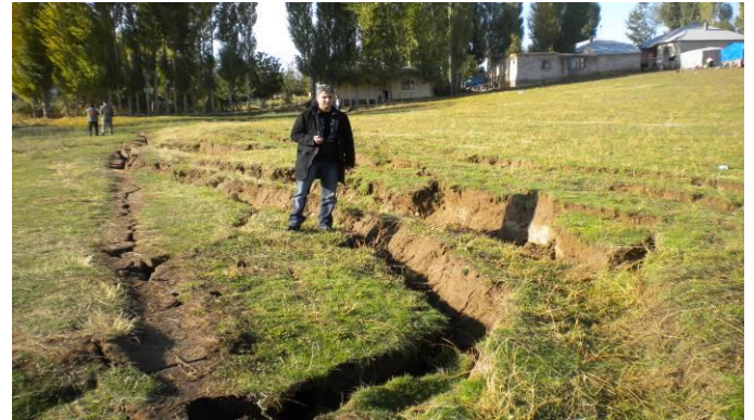
Fig. 4. Lateral spreading cracks in Celebibagi village (Ercis) affecting one-story masonry buildings at the background
