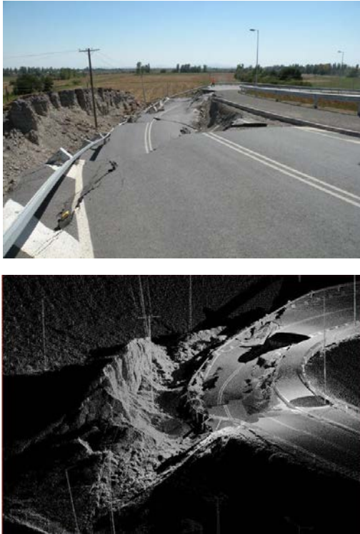
Fig. 3. Ground-based optical and LIDAR images of a failed overpass embankment on Ruta 5 as a result of the 2010 Chile Earthquake (courtesy of Kayen/GEER).
