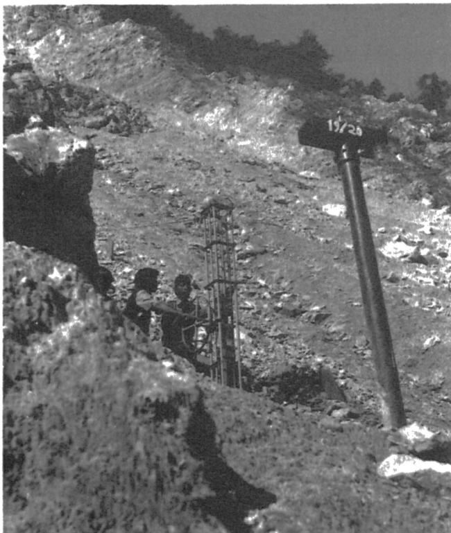
FIG. 9 - STITCHING OF COLLUVIUM ON THE SLOPE AT KALIASAUR BY A SIMPLE PILING MACHINE
