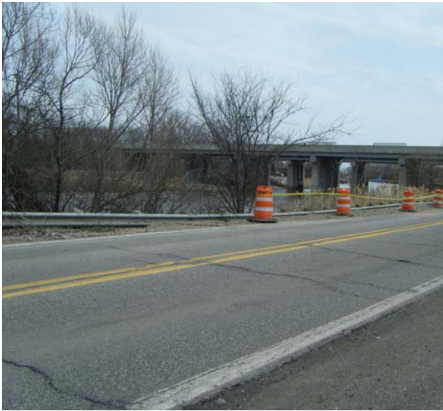
Figure 1: Photograph Showing dip in the guard rail along north side of South River Road.
