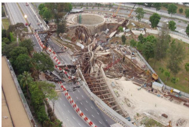
Plate 1. Photograph of the Collapse
