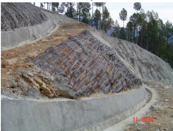
Fig.7-Slope stabilisation measures & construction of side drain on the benches in Crown Area
