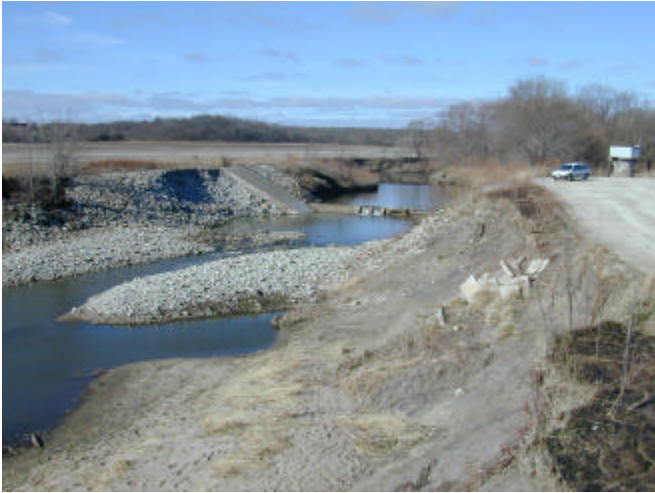
Fig. 2. Delaware River bank erosion
