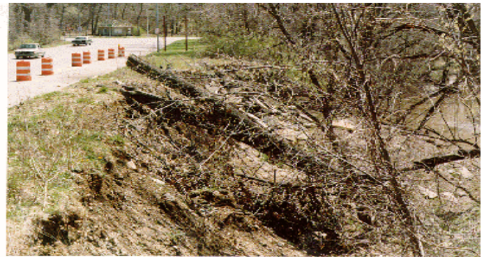
Fig. 1 BlueRiver slope failure prior repair
