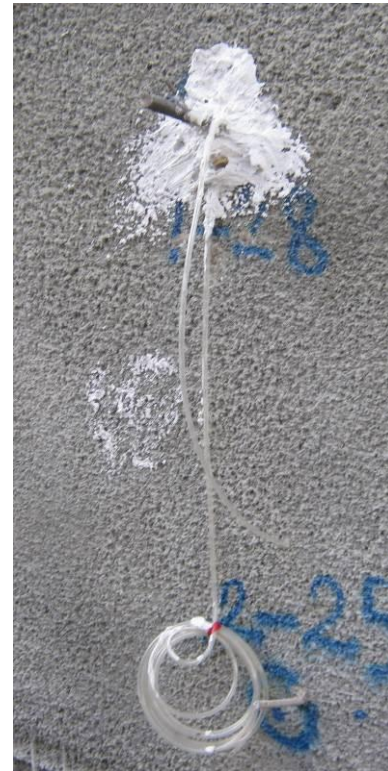
Fig. 10. Construction sequence: Installation of soil nails – insertion of nails into the drilled holes and preparing for injecting the grout
