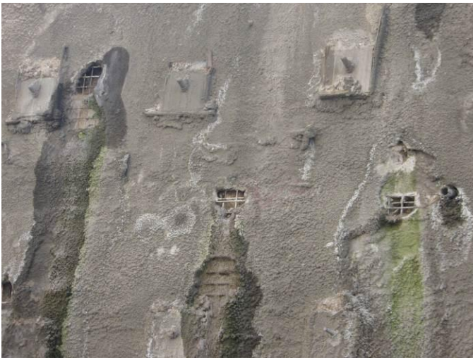
Fig. 27. Shotcrete scratched at the location of the water marks
