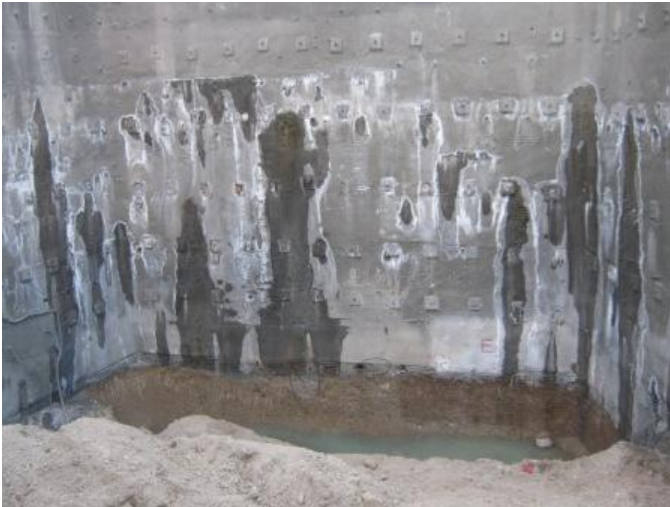
Fig. 26. Water marks on the surface of the E4 soil nail wall
