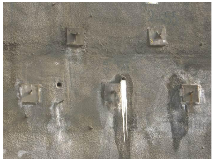
Fig. 29. Frozen water at the tip of a drain pipe installed on the soil nail wall (the drain was installed at this location after the water marks appeared on the shotcrete facing)
