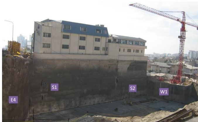
Fig. 17. S1, S2, E4, and W1 soil nail walls after excavation to the full depth
