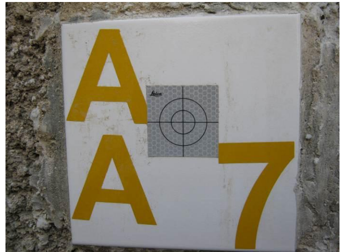
Fig. 24. Target installed on the shotcrete facing Recording of the deformations of the soil nail walls was continued until 14 th of June 2010 well after the excavation process was completed.
