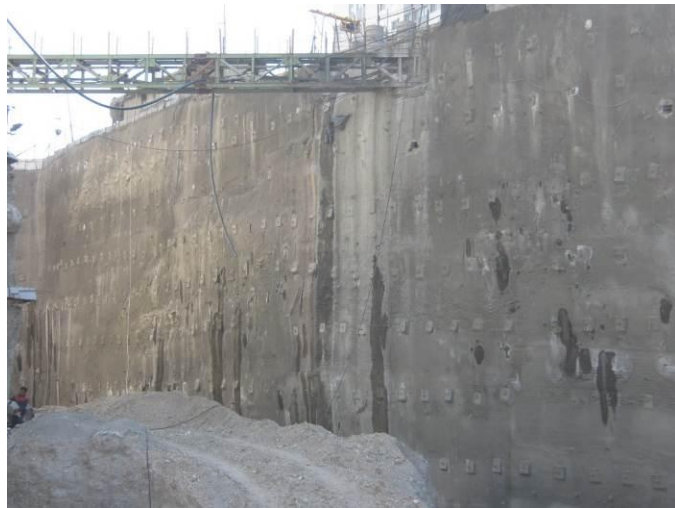
Fig. 31. Strut holding the gas pipe between the E3 soil nail wall and the TOOBA tower
