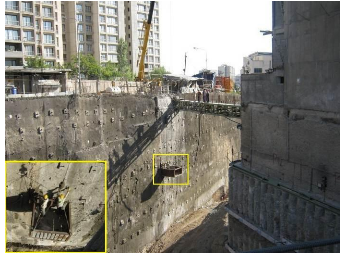
Fig. 34. Workers installing the drains on the locations where water marks have appeared on the surface of the shotcrete
