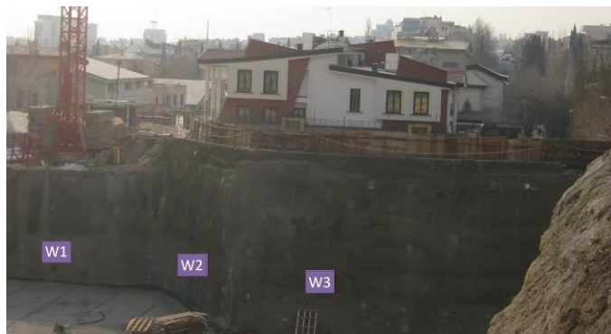
Fig. 18. W1, W2, W3 soil nail walls after excavation to the full depth
