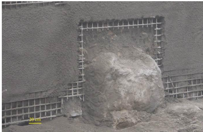
Fig. 4. The site consists of silty and clayey sand and gravel along with boulders up to few meters in diameter
