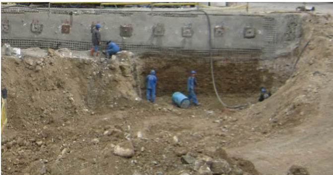
Fig. 13. Excavation for the soil nail walls in blocks rather than lifts at some locations for increased stability
