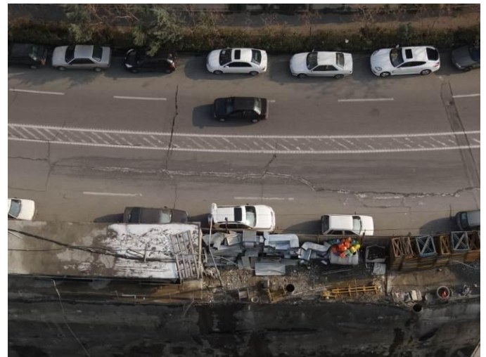
Fig. 35. View of the crack at the surface of the tarmac captured from the roof top of the TOOBA tower
