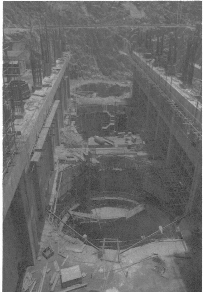
Fig. 4 Photo showing shafts
