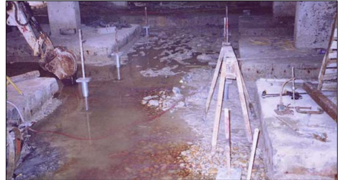
Photograph E – Rock anchor head assemblies
