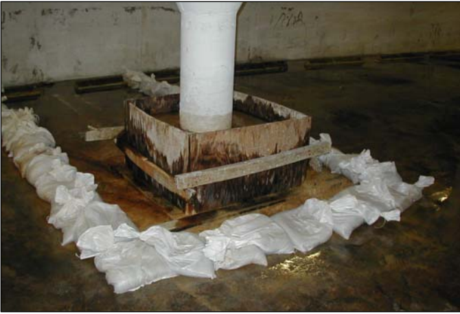
Photograph D – Observed seepage within subterranean level
