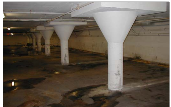
Photograph C – Observed seepage within subterranean level
