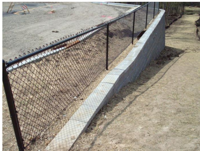
Fig. 7. Subsidence of facing blocks along north side of retaining wall (view is opposite that shown by Fig. 1).
