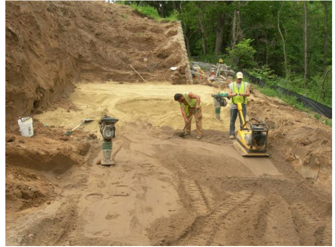
Fig. 13. Clean sand capped with well-graded crushed limestone aggregate base material across the entire base of the MSE wall.
