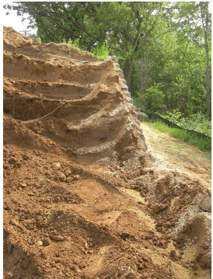
Fig. 11. Wall partially deconstructed, with relative lack of drainage aggregate and no horizontal drain tile or geotextile filter fabric observed.
