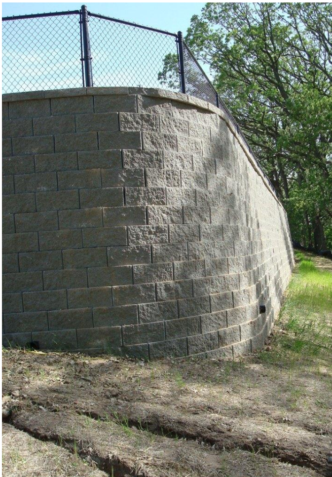
Fig. 5. View looking south from northwest corner of wall, showing drain pipes located above bottom-of-wall, and bend along west line of wall. Surface erosion due to overtopping of wall is present in foreground.
