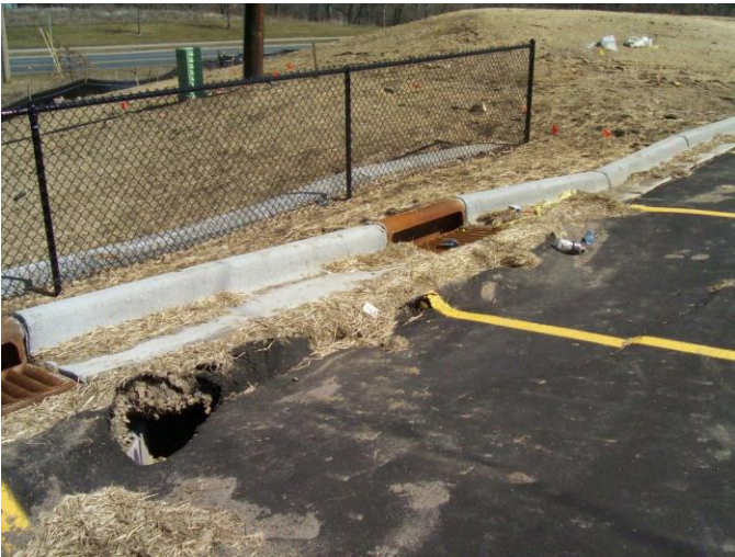
Fig. 3. Subsidence and openings in pavement near catch basins located within wall backfill. Settlement of the wall facing blocks (behind chain-link fence) is also apparent.
