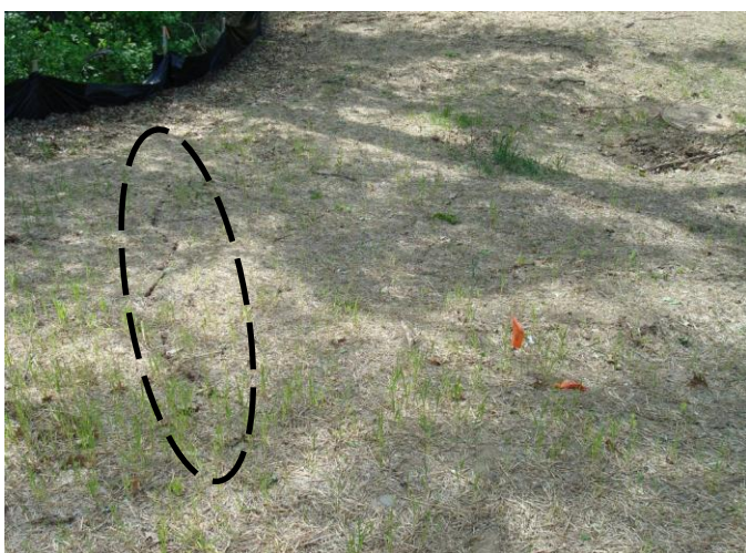
Fig. 6. Surface crack along south (lefthand) edge of backfilled storm sewer trench.
