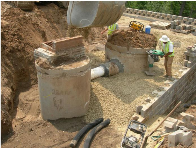
Fig. 15. Compacting gravel backfill around catch basin risers. Geotextile-wrapped filtered drain tile is also visible.
