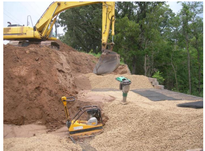
Fig. 14. The reconstructed MSE wall was backfilled with a well-graded gravel filter material, with a three-foot wide well-graded sand filter zone behind.
