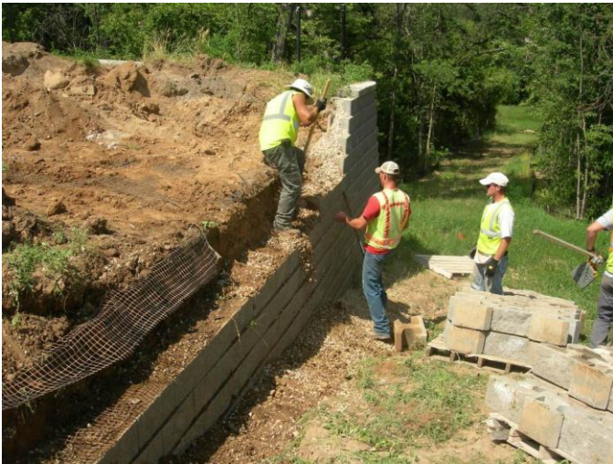
Fig. 10. Early stage of MSE wall deconstruction. Note drainage aggregate within blocks, but not extending 12 inches behind facing blocks per design.
