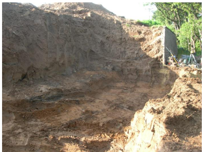
Fig. 12. Overexcavation was performed below bottom-of-wall elevation, based on field judgment (and field density test results) showing marginal density of in-place fill soils.
