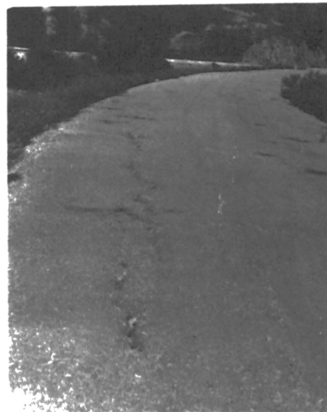
Fig. 1. Longitudinal cracks on the embankment.
