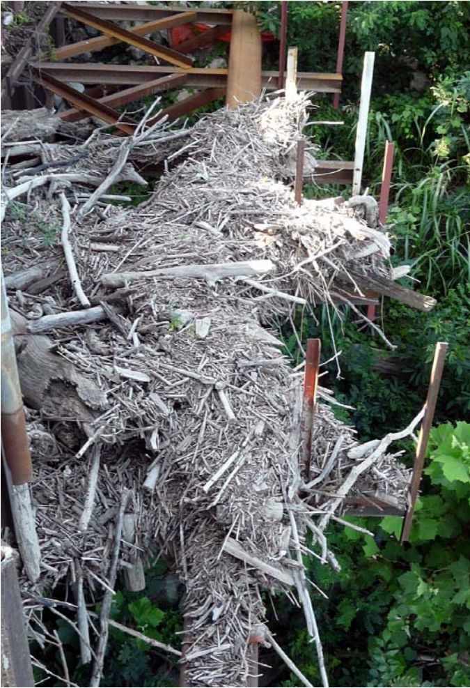
Fig. 13. Debris on tension bar protective structural tube.
