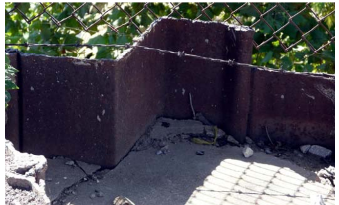
Fig. 6. Settlement of existing access roadway cap.
