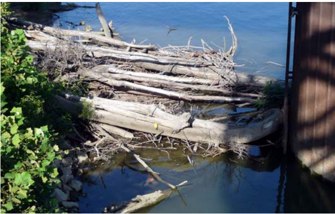
Fig. 14. Debris at mooring cell upstream of load platform cell.
