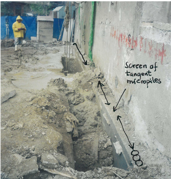
Photo 4. The screen of tangent micropiles position and the beginning of slurry wall execution near the old building
