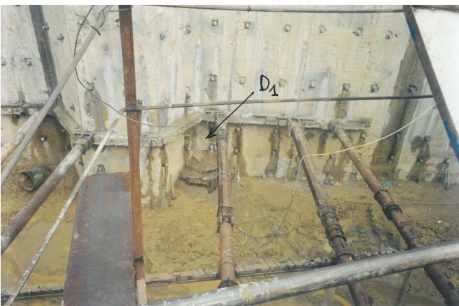
Photo 8. Slurry wall defect situated adjacent to Armenian library at 16 m deep (D1 on the figure no 3)
