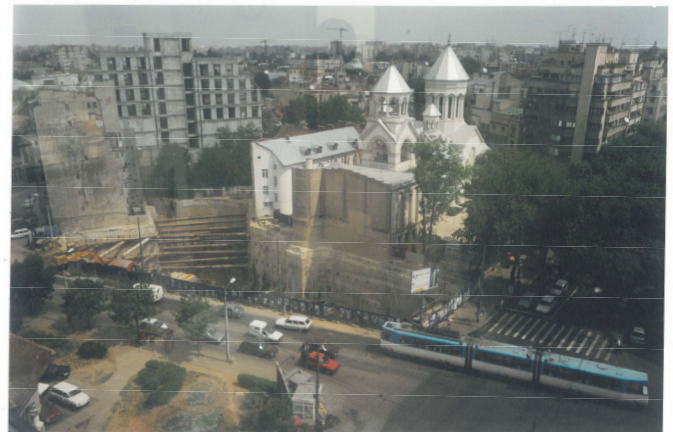
Photo 1. General view of the "Armenian complex" and of the deep excavation area
