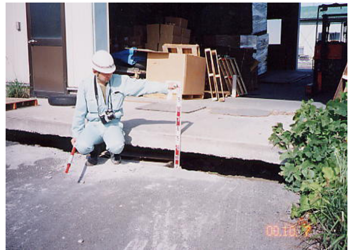
Photo 4. Ground subsidence at an industry in Takenouchi industrial park
