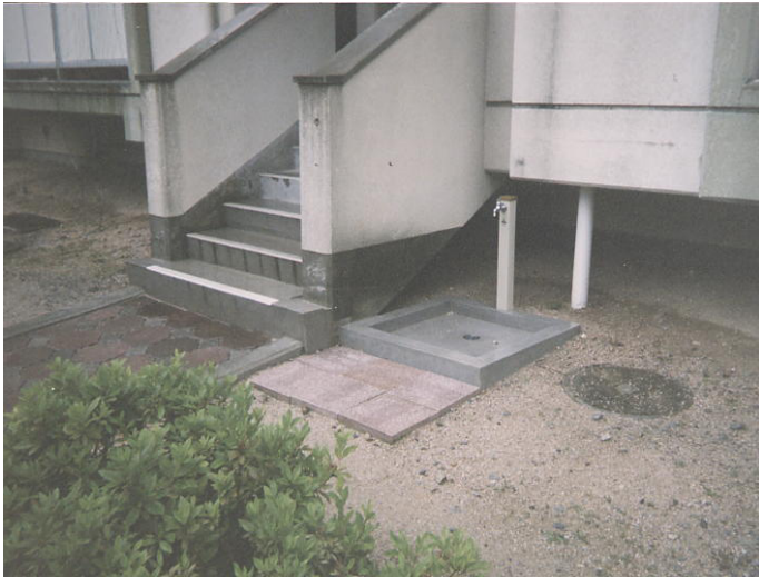
Photo 7. Evidence of ground subsidence due to earthquake observed around pile-supported apartment
