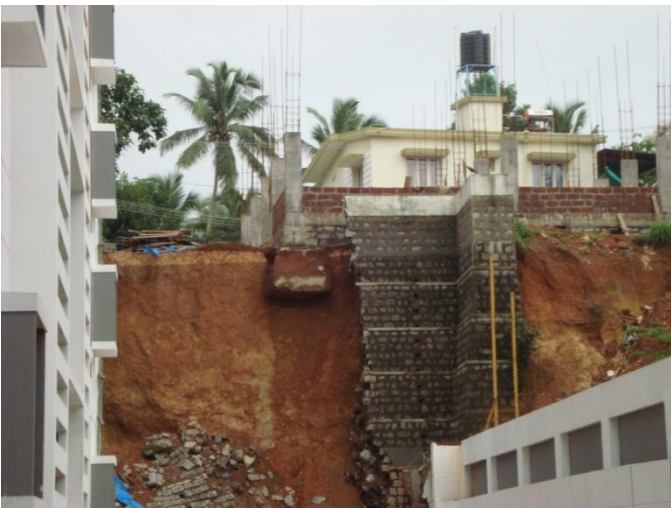
Fig.13. Another failed (so-called) masonry retaining wall
