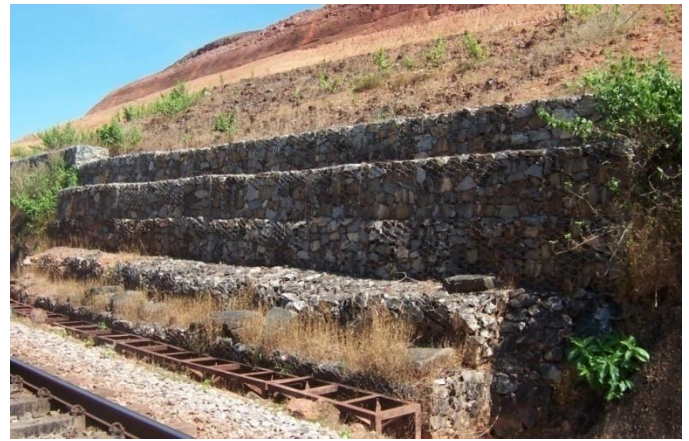
Fig. 11. A gabion toe retaining wall on the Konkan railway stretch using hexagonal wire meshes
