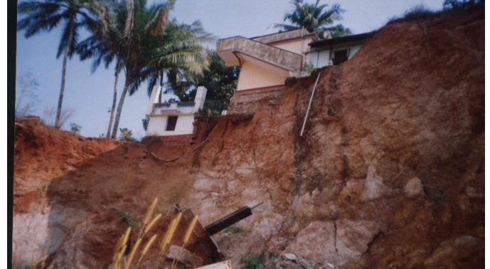
Fig.8. Adjacent structures endangered due to excavation
