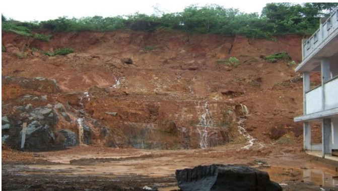
Fig.7. Excavation changing drainage pattern and endangering stability of excavated slope
