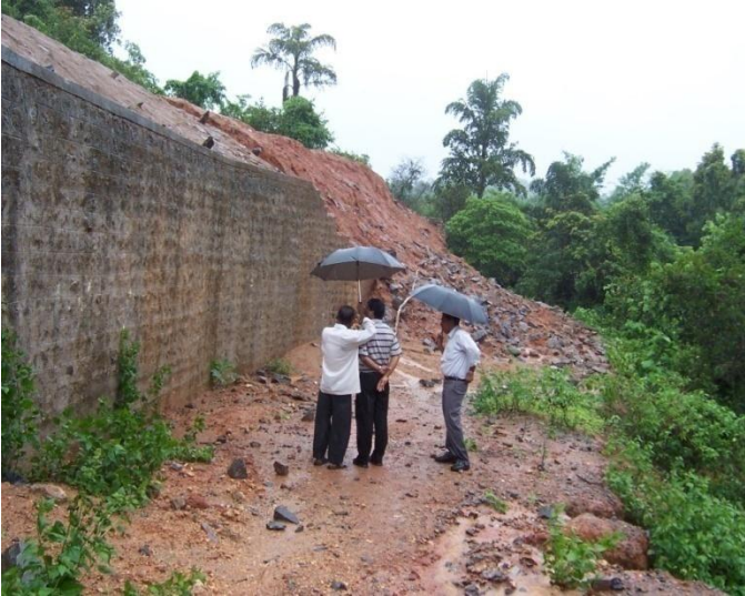
Fig.12. A failed masonry retaining wall (cosmetic wall) due to under-design
