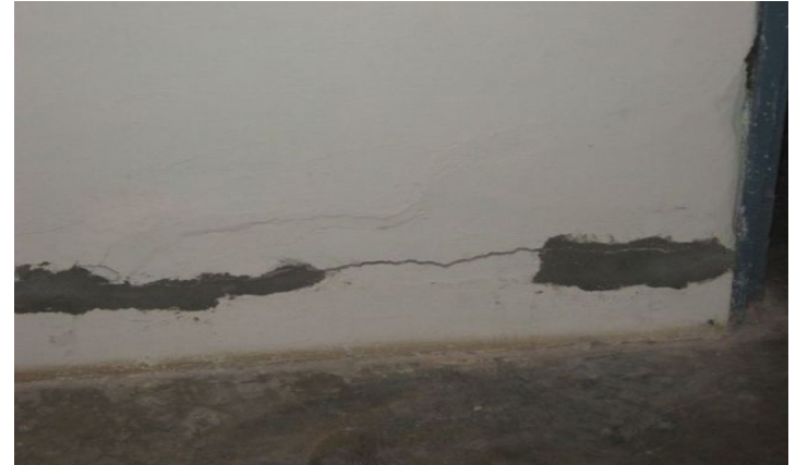
Fig.3. Damaged wall of bedroom
